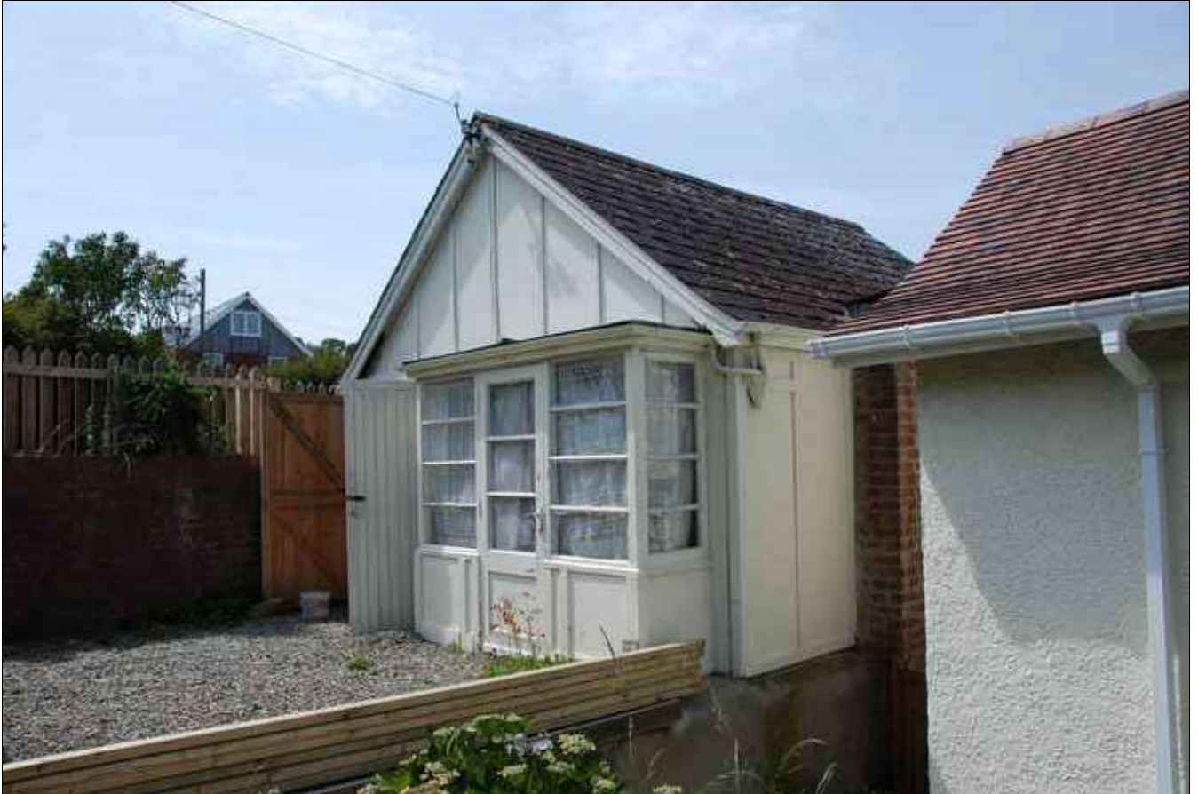
The Chalet ... in the throes of renovation ... situated to one side of the Main Residence
